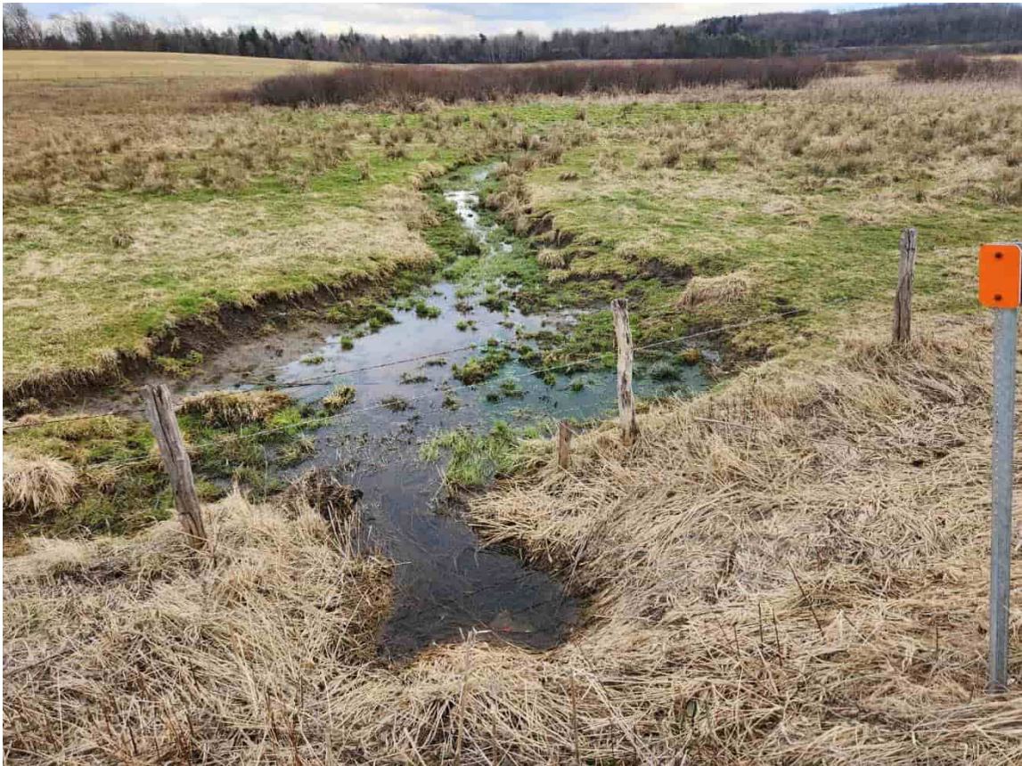
Photograph of existing conditions and lack of positive drainage upstream of culvert MR-3
